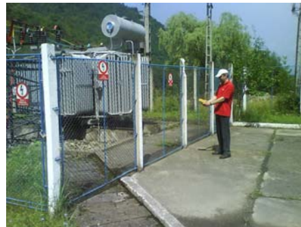
Fig. 8. Measurement of low-frequency magnetic fields in the proximity of a power transformer.
