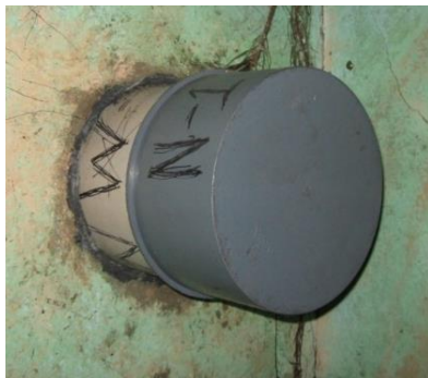
Fig. 2. Can on bare walls.
